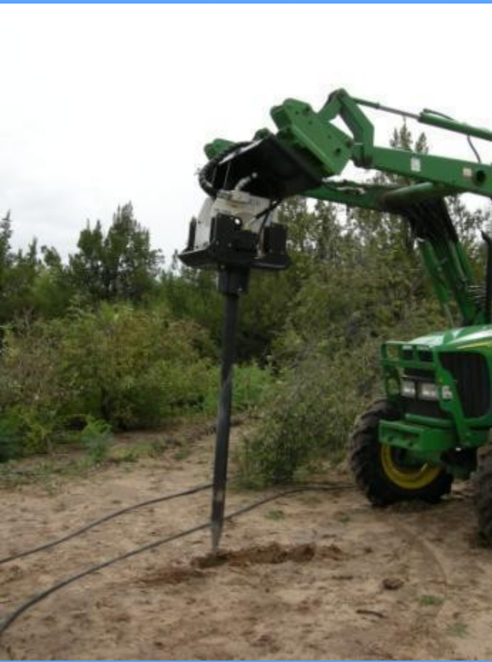
Hydraulic compactor with stinger (3.5-inch diameter) attached to the loader of a 65-hp farm tractor
